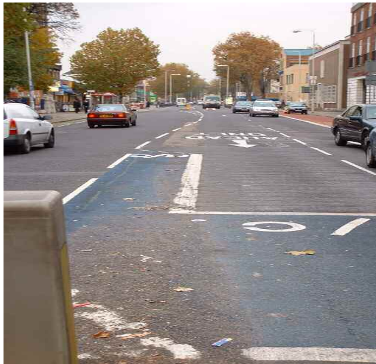
Photograph 6: Build up of grit and debris in the motorcycle filter lane
