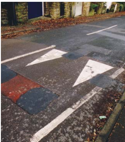
Poorly reinstated traffic calming. Keith Sharples Photography.
