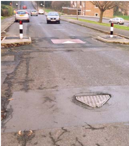
Poorly reinstated traffic calming. Keith Sharples Photography.
