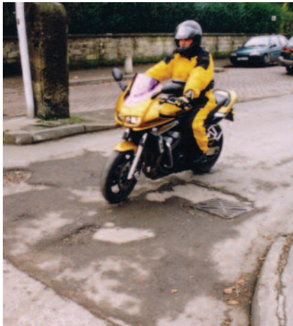
Potholes present a particular hazard to motorcycles. Keith Sharples Photography.
